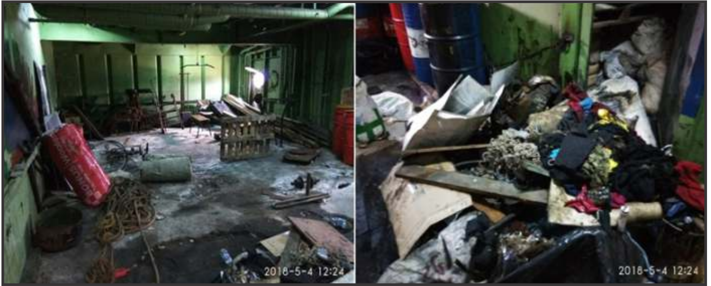
Gymnasium space is appeared to be suffered with fire accident in the past and accumulated with garbage
